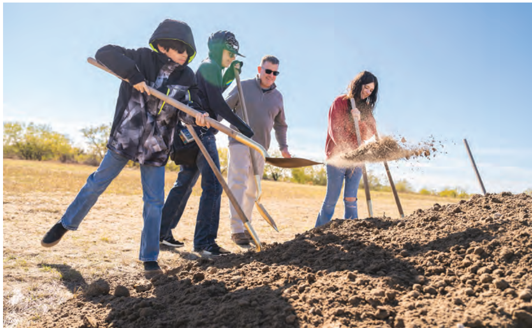
Parishioners join in breaking ground at St. Teresa of Calcutta Parish in Roanoke for the construction of a parish hall that will house the fast-growing parish community. (NTC/Juan Guajardo)
